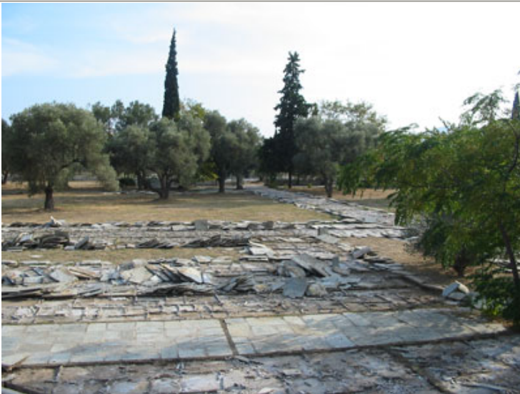
The whole place is being re-tiled and generally renovated as the 2004 Olympics approach
